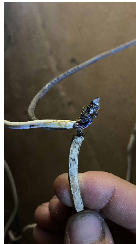
One of the substandard wiring crimps
